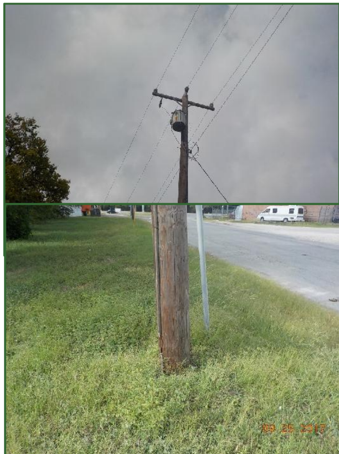
PHOTOGRAPH #8 and 9 – Unmarked transformer and vegetation at the base of the pole on the Site.
